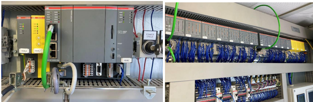
Figure 3 ERTG ABB PLC assembly on E-room including the remote I/O used for the pilot testing phase.
