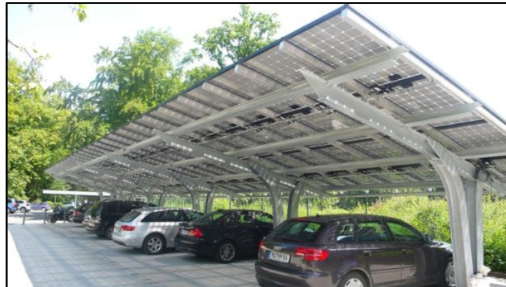
Fig. 3. Solar PV panels On top of Parking Lots
