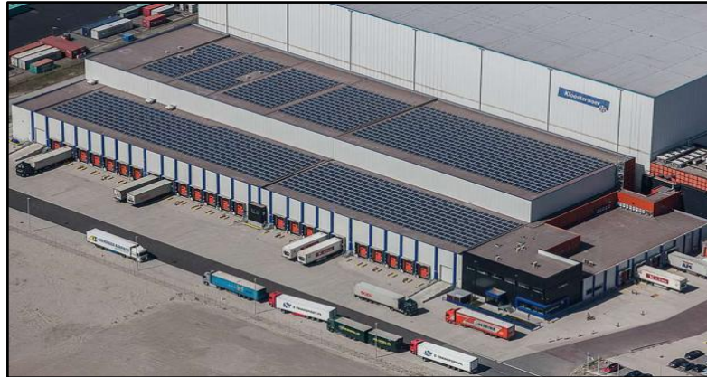
Fig. 1. Solar PV panels on the roof of warehouses and cold storage facilities
