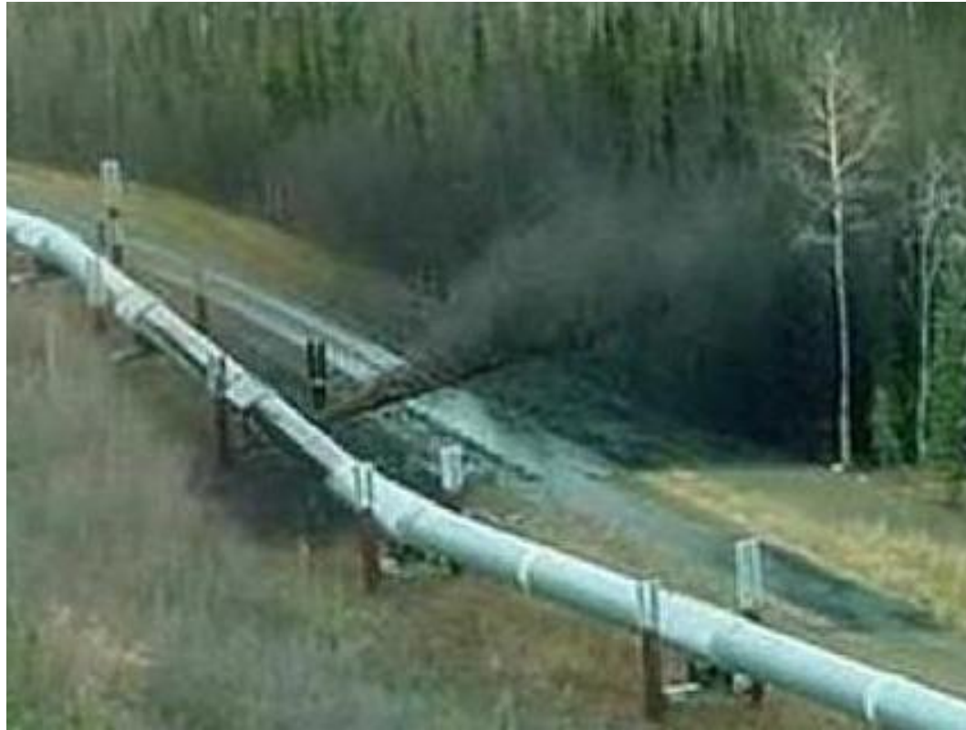
Fig.2. Pipeline leakage in Alberta Canada
