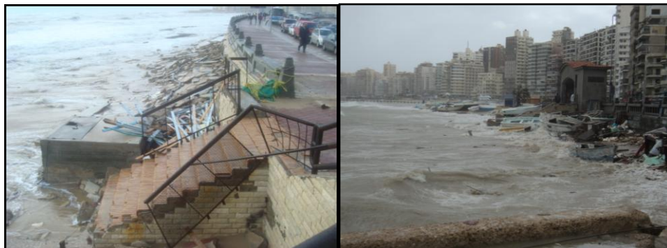
Figure 17: Damages of Sidi Beshher beach due to waves attacks during 2010 storm.
