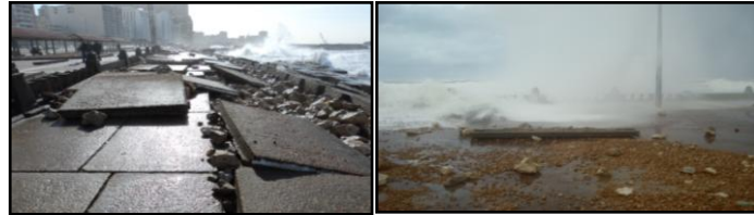
Figure 16: Damages of the side walk and concrete fences at Loran area.
